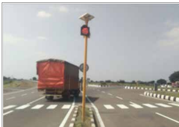
Solar blinker sign at Black spot No. MH-009
